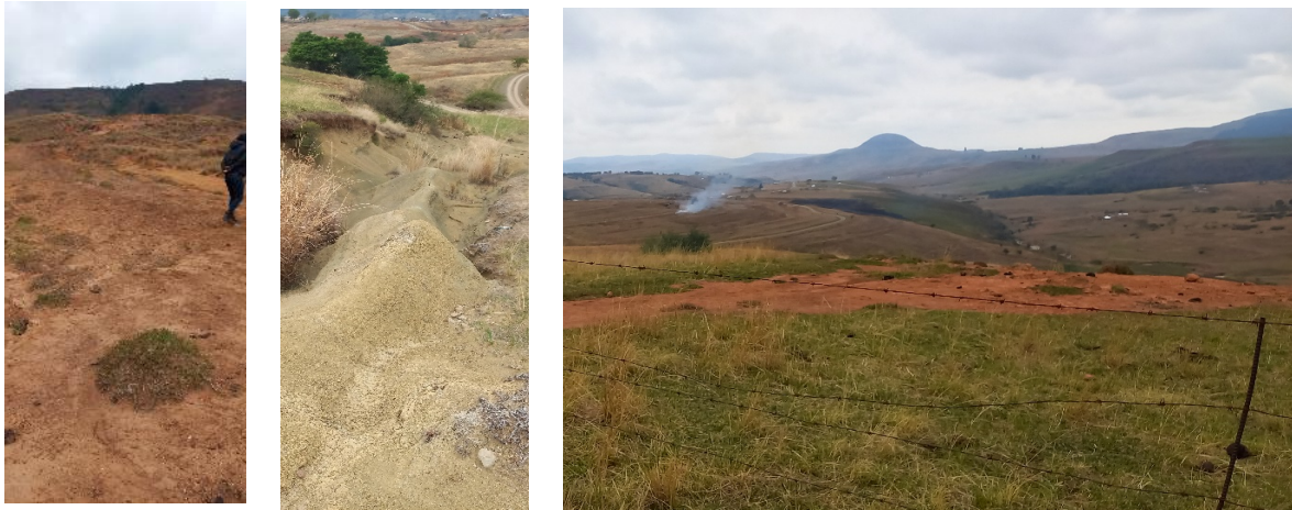
Figure 3: Above Left to Right: Views of the extensive erosion of the ‘cattle paths’ above the road, and past the dip tank. The picture on the right shows the top of the small hill, just beyond the fence where the erosion control works should start.
