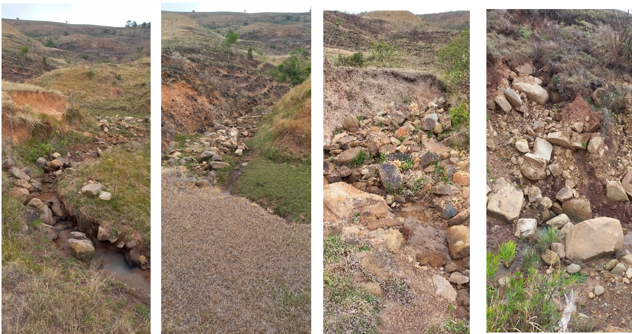
4, eroding side walls which are very unstable in some sections.
