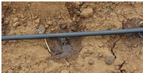
A well functioning string dripper that makes a wetted circle around the dripper
