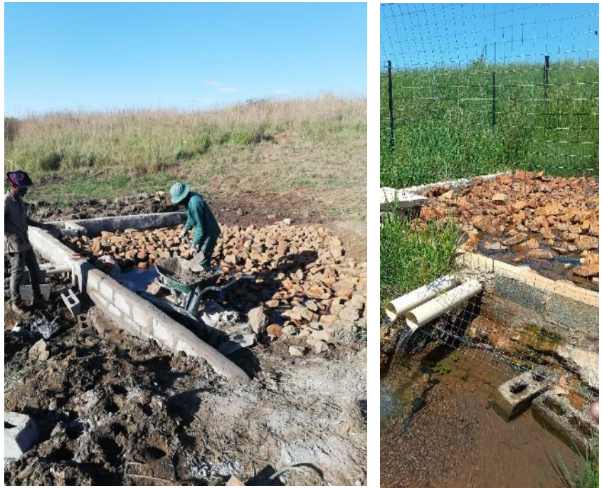
Figure 25: Below Left and Right: The 2 x5000l header tanks at installation and recently in Feb '23 – also fenced.
