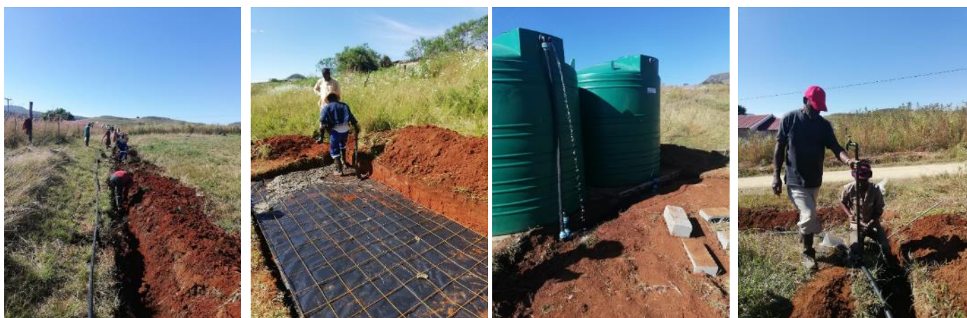
Above left to right: Laying of pipe after digging ditches. Building of JoJo tank platform. Connecting of the two JoJo tanks and linking to the spring. Water is flowing. Constructing the 4 taps in the line.
