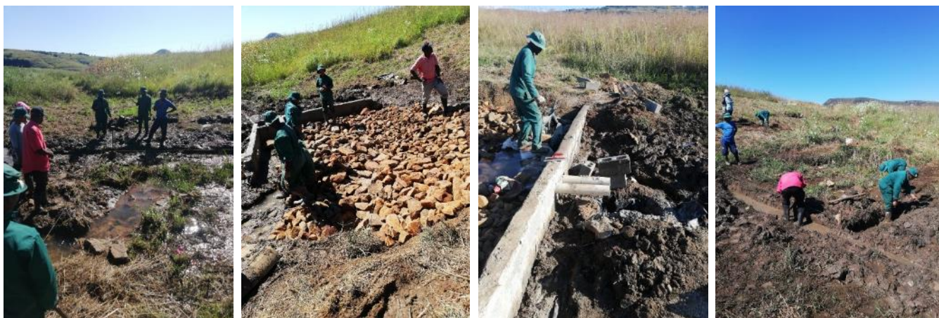
Above Left to Right: Pegging the position of the v-box wall with Chris Ndlela (red shirt). Covering the area with collected rocks and building of the corner collection box and corner of the wall. Finalisation of the wall with the two outlet pipes for local water access. Digging the ditches for mainline pipe.
