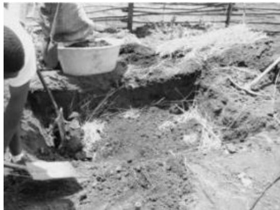
A trench bed in Potshini being filled and mixed. Here the top soil is being added back into the trench Notice the yellow subsoil on the one side. It is not being used.
