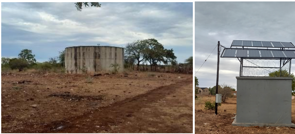
Figure 9: A view of the 700 000l village header tank in Mayephu and one of the boreholes supplying this tank fitted with electricity from both a power line and solar panels, for dual supply.
