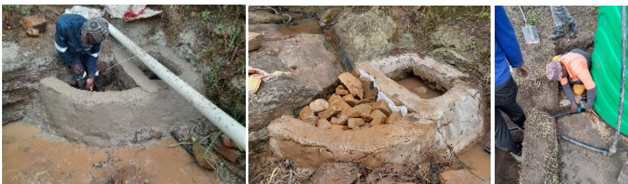
Figure 20: Above Left to right: Construction of the weir and v-box in stream for both Sections A and B. The finalised weir, with shade cloth and rocks in the inlet chamber and the brake pressure tank 92500l), with pipes connected from the source and towards the header tank – also for both sections A and B.
