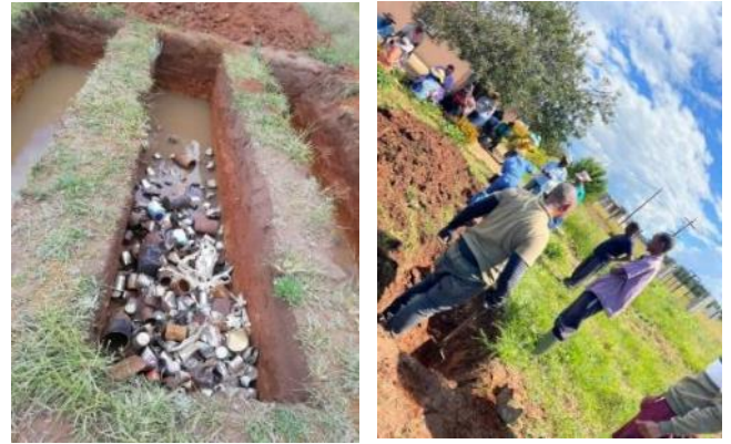
Figure 10: Right and Far Right: Mr Potlo and the Mechachaneng learning group members work on digging the trench beds and filling the bottom with used tins, prior to further collection of organic materials.
