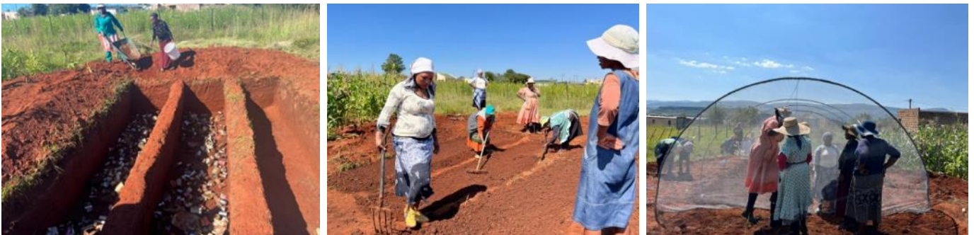
Figure 9: Above Left to right: Construction and filling of trench beds, prior to construction of the tunnel by the CRA learning group members in Nchodu, at Phumla Nyembezi's homestead.
