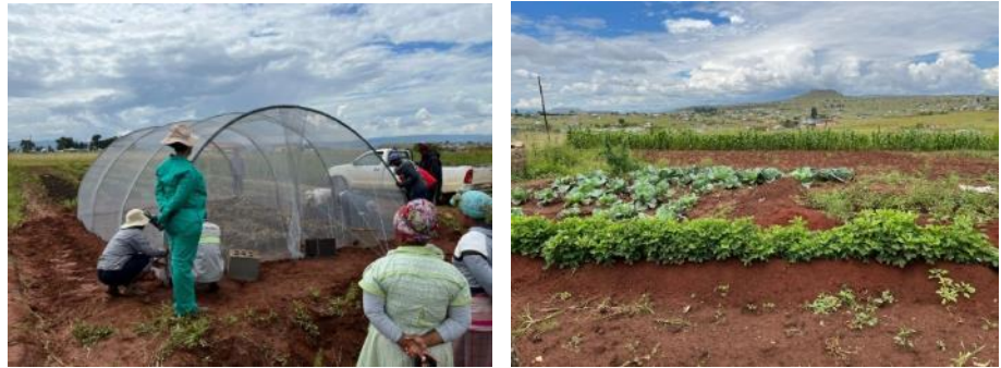
Figure 13: Right and far right: John Tefani's tunnel under construction and a view of his garden, with his maize field in the background.
