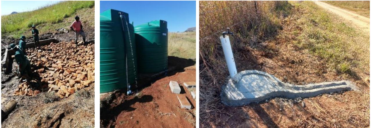
Figure 22: Above Left to Right: The v-box under construction for protection of the spring. The two header tanks installed and connected to the spring – they have filled up and water is flowing, and one of the 4 taps installed for the 23 households to collect water from. All households are within 200-400 m of a tap.
