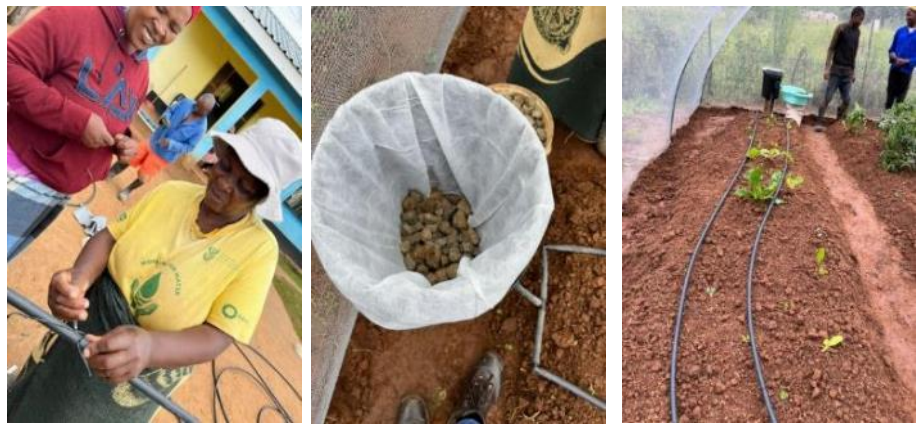
Figure 14: Right Nkau: Two group members putting the small spaghetti lines into the drip pipe – the drippers. The bucket with it's gravel and sand filter for use of grey water and the drip kit installed on one bed in a tunnel.
