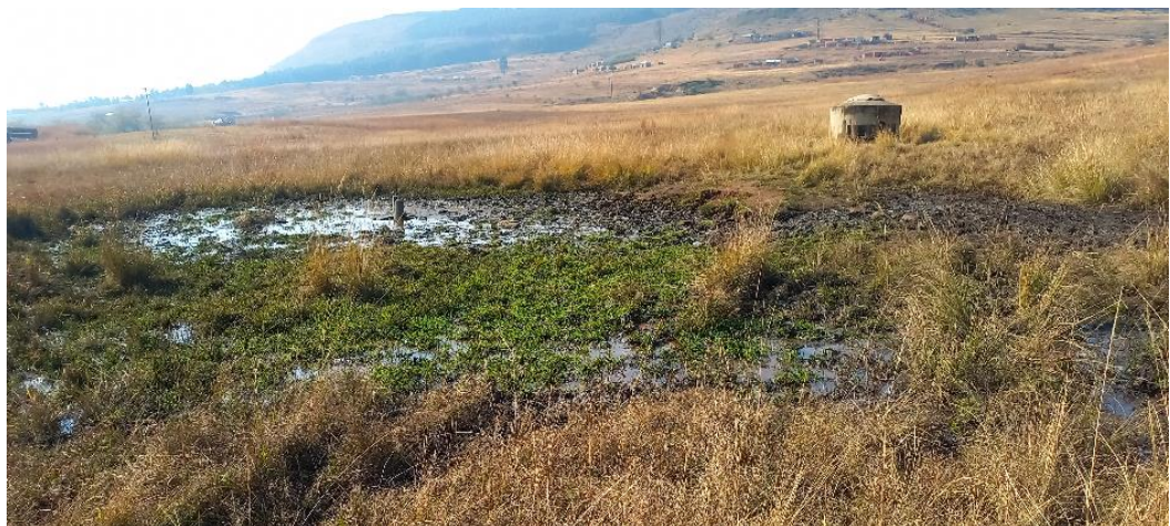
Figure 7: The old, protected spring with leaking header tank and inaccessible tap.
