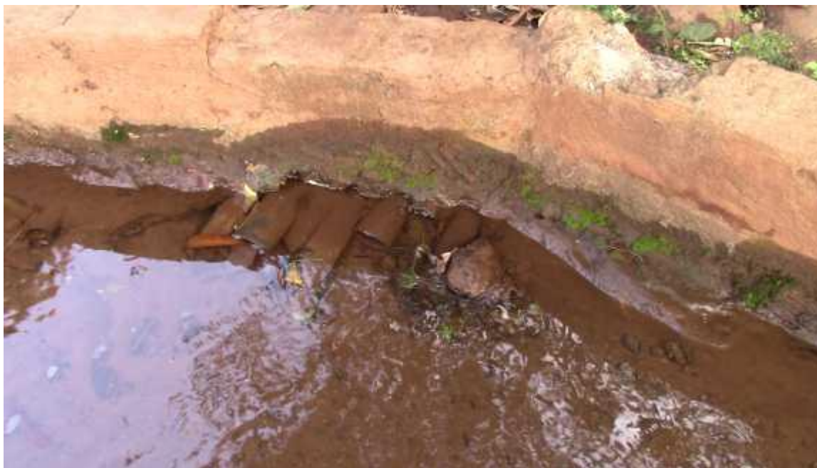
Above: One of the sites where pipes are placed in the furrow.
