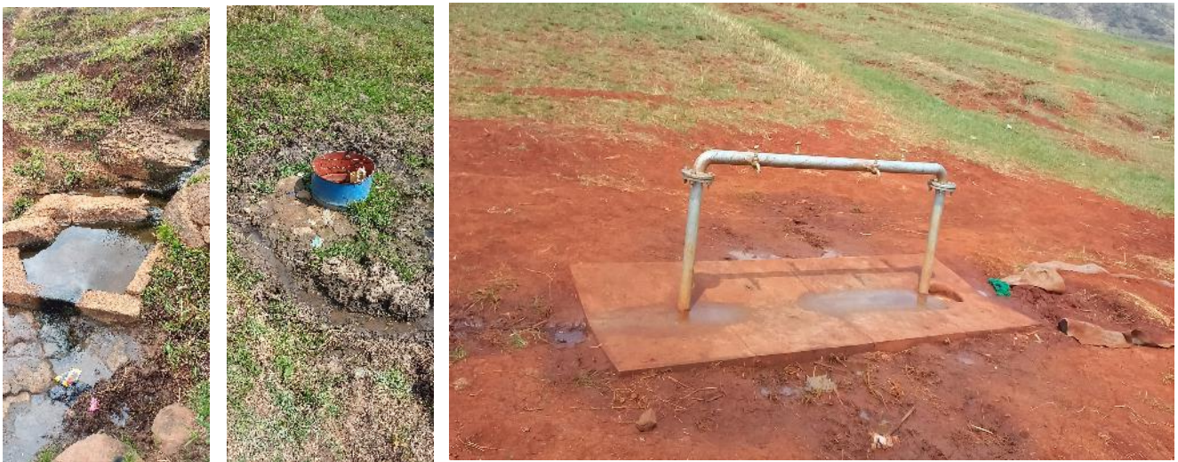
Figure 7: Above left to right: Protected springs by local community members and the taps provided by the Municipality for a borehole drilled directly into the wetland.
