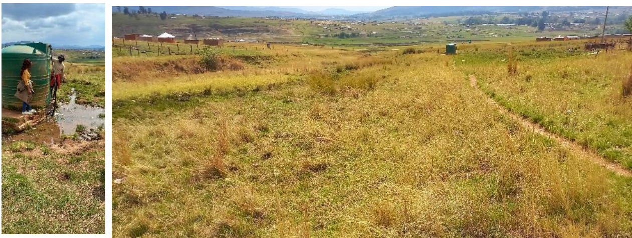
Figure 8: An old spring protection point with a JoJo tank that was installed before 2000. The tank is leaking, and the overflow pipe was removed, creating a small pond in the area where water should be collected. In addition, the tank is on the edge of one of the homesteads on the edge of the wetland and there have been 'ownership' issues both of this water and of the wetland as a result.
