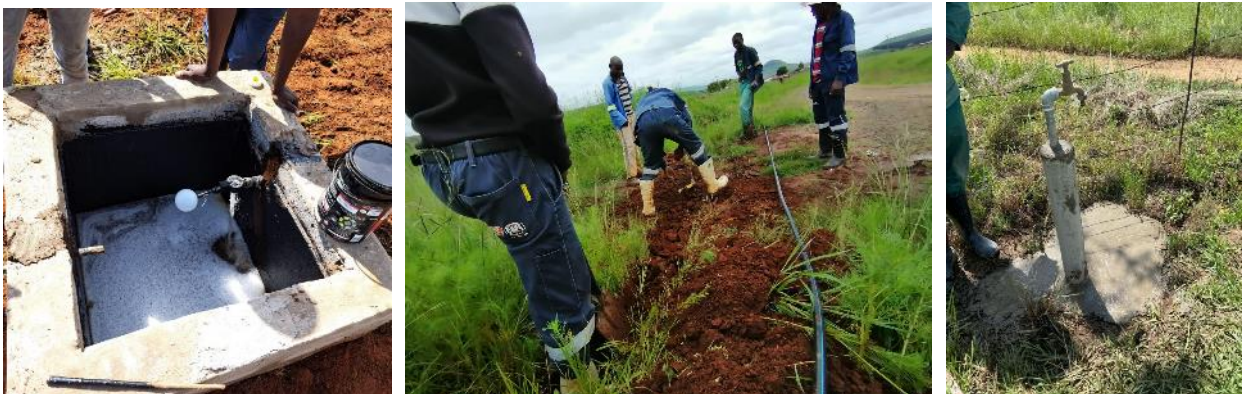
Figure 7: Above left to right: The Village A break pressure tank, installing pipes and an example of one of the 15 taps installed.
