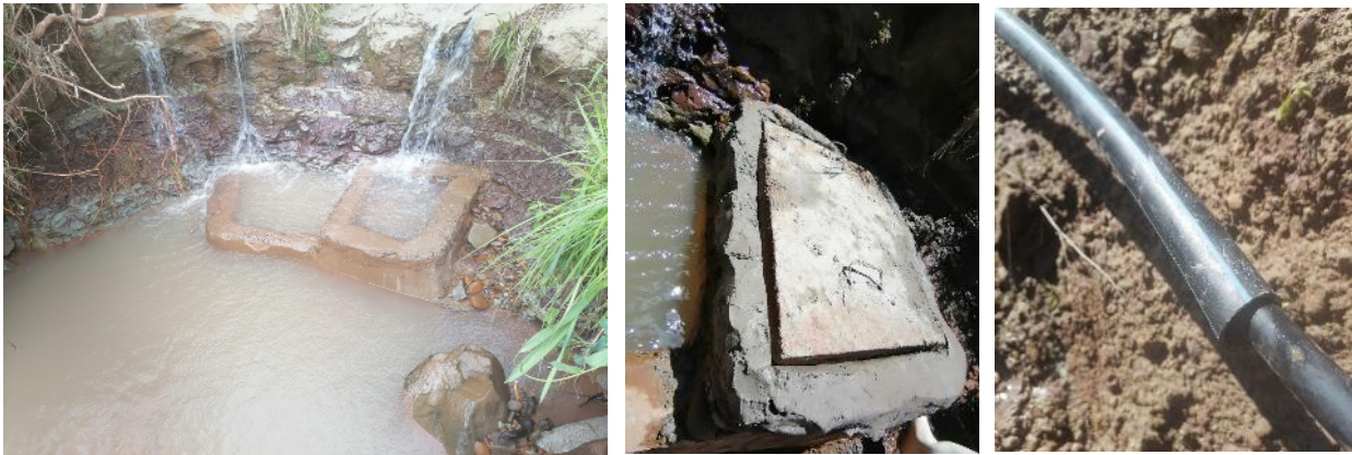
Figure 6: Above left to right> A view of the flooded source, the v-box lid now anchored with an additional layer of masonry and hard piping sleeves added for vulnerable piping, which cannot be buried due to rocky streambed conditions.
