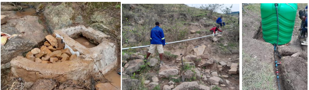
Figure 5: Above left to right: the source development consisting of a settling chamber and v-box in stream, the rigid carbon steel piping installed to cross the gullies and installation of the break pressure tanks.
