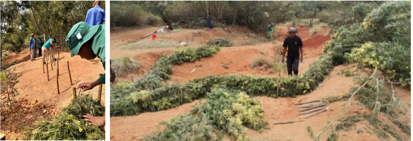
Figure 18: Above Left and Right: Constructing a brush pack and a view of one full brush pack constructed across the gully. Note that the line for the brush pack is roughly a half-moon shape along the contour.
