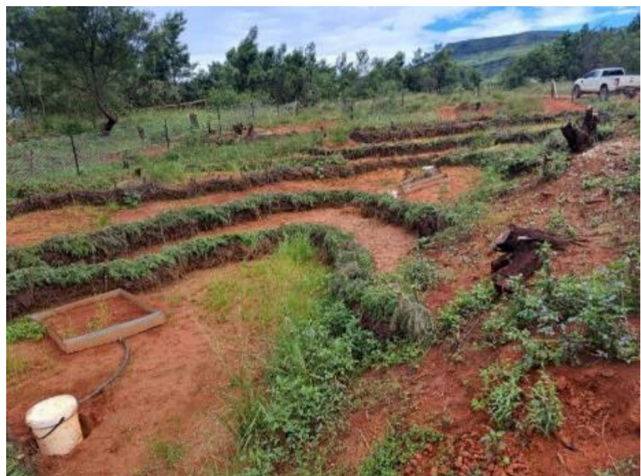
Figure 20: Right; A view of the new brush packs that were built, both over the 1 st set which had been covered by sediment and in-between the initial brush packs to allow for further sedimentation and re-seeding of grass. In the foreground is one of the run-off pans that were placed throughout the site to measure run-off.
