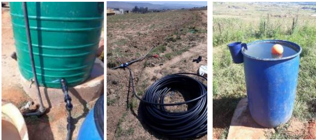
Figure 29: Above Left to right: the 2200L header tank from which water is gravity fed to 9 households. The piping being installed leading to the households. The 200L drum with float valve installed at each household.
