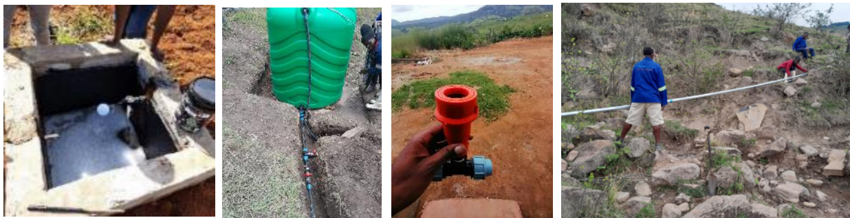
Figure 35: Above Left to Right: A brake pressure tank with float valve under construction. One of the header tanks. An example of an air valve for further air and pressure release. A section of carbon-steel piping in a portion where pipes could not be buried.
