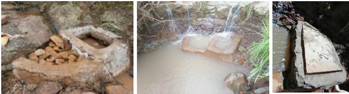
Figure 34: Above Left to right: the intake and silt chambers built into a small mountain stream in the dry season. A view of these small structures in the rainy season. The cement lid for the 2 nd chamber to only allow 'cleaner' water from the initial intake chamber to pass through to the tanks.
