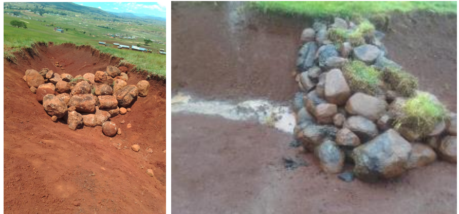
Figure 23: Right and far Right: Community level efforts in a village in the Northern Drakensberg to do gully restoration. This structure was quite stable due to it's size and also the size of the rocks used, but was not well constructed and not keyed into the banks – making it vulnerable to further erosion.
