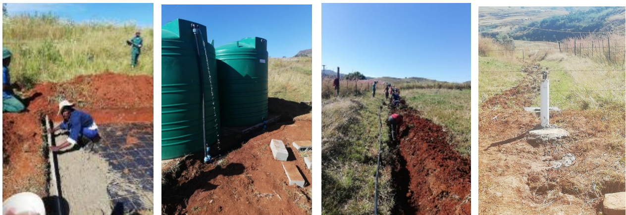
Figure 33: Above Left to right: Construction of the cement platform for the tanks. The two joined 2500l JoJo tanks. Digging ditches and laying pipes for the community taps. An example of a community tap upon completion.
