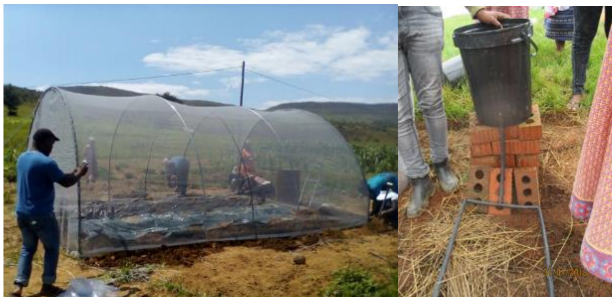
Above Left: One of the 4-6m tunnels completed by community members. Black plastic has been used to temporarily cover the three long trench beds constructed inside the tunnel. Above right: One of the drip kits set up outside the tunnel (another is inside for comparative purposes).
