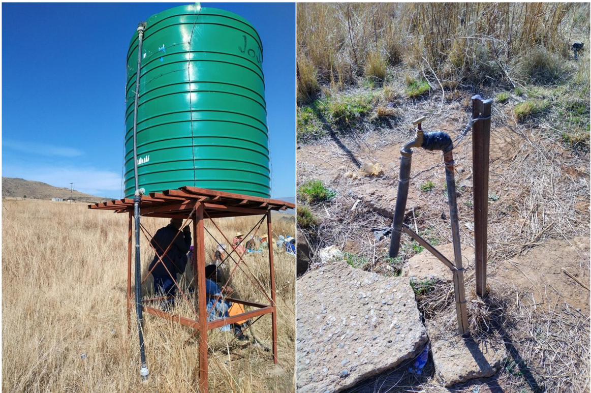
Figs 3 & 4: 5000l water tank and standpipe fed by borehole
