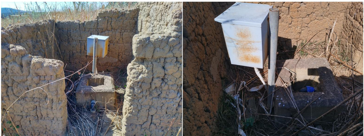
Figs 5 & 6: Borehole and control box
