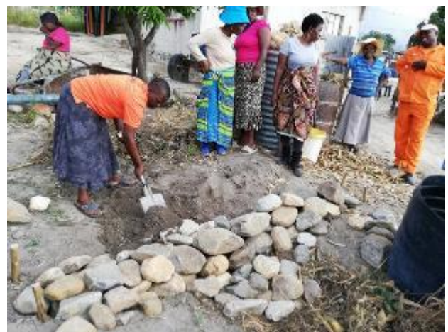
Figure 34: Right: Putting in the final completion touches to a check dam built across a gully forming at the top end of the garden/field
