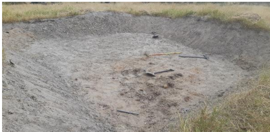
Figure 39: Right; Esinah's dam after the bentonite was worked into the walls and floor of the pond
