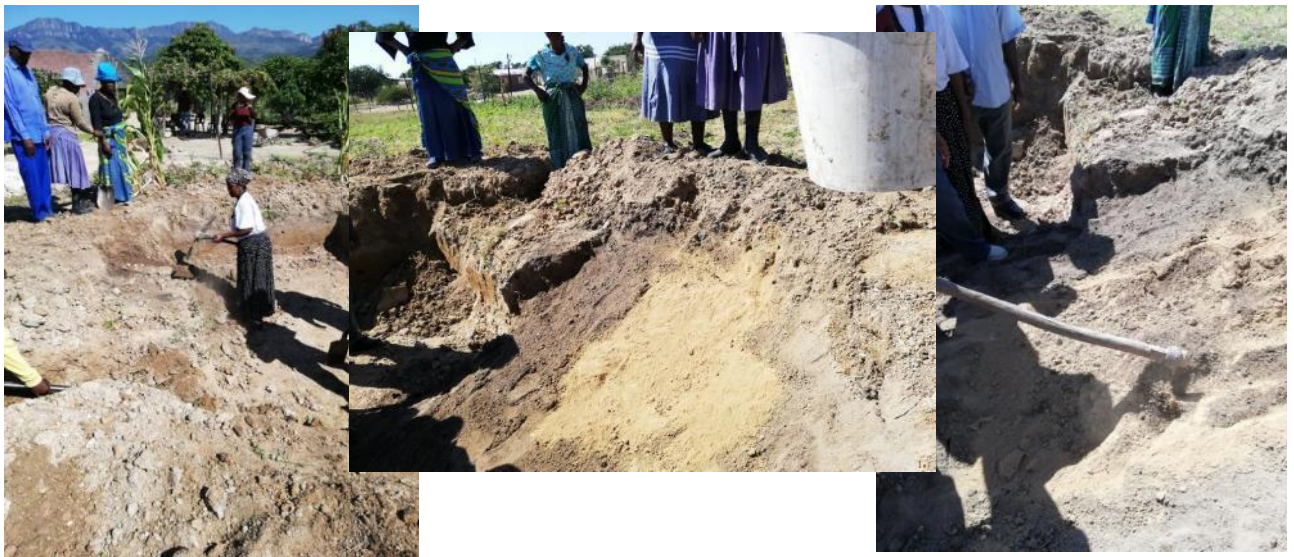
Figure 37: Above left to right: Measuring out a circle – to change the dam shape from a rectangle and then shaving the perpendicular walls to be at an angle of roughly 35 degrees. Marking out a m 2 area and then evenly distributing 12,5 kg of bentonite over the are and carefully mixing in the bentonite into the top 10cm of the soil on the bank
