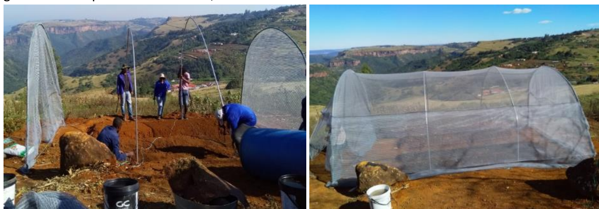
Figure 3: Tunnel construction. Left; the placement of the arches and Right; pulling the netting over the arches to create the shade cloth structure.
