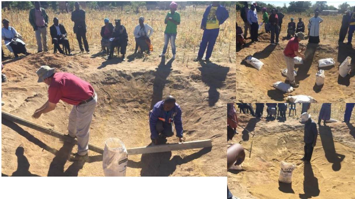
Figure 41: Left, marking out grids, top right; bags placed on grids & bottom right, bentonite spread.
