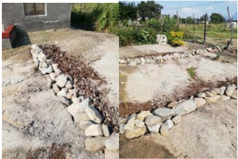
Figure 33: Right: A stone line constructed as close as possible to the top of a slope as a starting point, note that it is keyed in and “slants” slightly uphill. Manure has been worked into the soil above the stone line, for planting. Far Right: Two stone lines constructed around 2 meters apart and planted to Sesbania sesban seedlings
