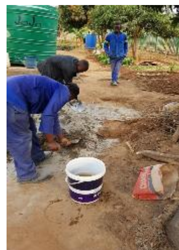
Right: Israel and Noah, the local builders assisting Eric (in this picture busy mixing cement). Noah was one of the young men who wanted to learn to do the construction. He had very little previous experience. Israel's help was invaluable and he would be able to continue into the future to construct similar tanks without much supervision. Eric is employed by Southern Irrigation as a master builder and has years of experience building these tanks.
