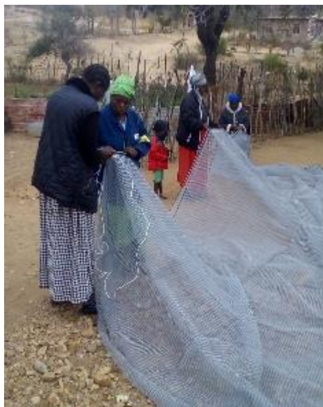
Far left: Mariam Malepe fixing the tunnel door panels and Left: Christina and Norah sewing the nets/panels of shade cloth together
