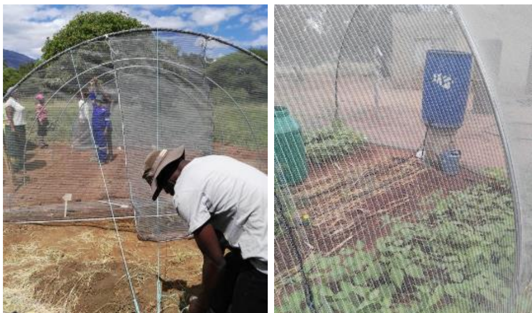
Figure 11 Left: A group of participants from The Oaks and Lepelle construct a tunnel together. Right: A working tunnel in Sedawa, where a drip kit has also been installed and crops are planted in trench beds. Mulching is in evidence.
