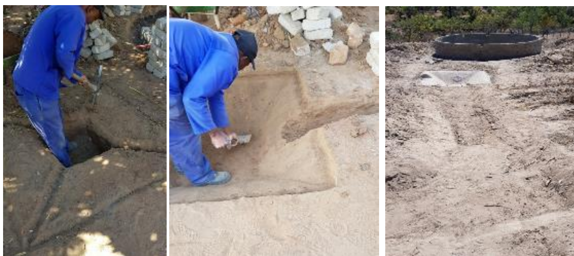
Above left and middle: Eric from Southern Irrigation carefully digging out the silt trap. Right: A view showing the inlet furrow in the foreground of the picture, the silt trap in the middle and the overflow furrow from the silt trap moving downslope to the left of the tank.
