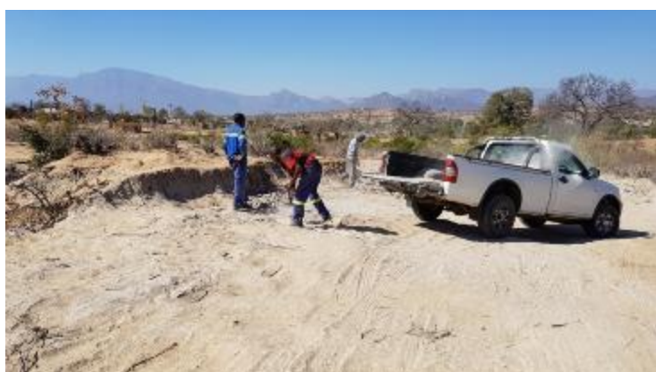
Left: Collecting sand for the building process - now being done by the construction team. A vehicle had to be hired for the purpose.
