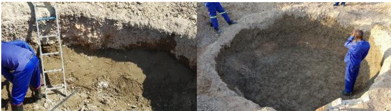
Above left and right; Views of the corrective plastering that needed to be done at Norah Mahlaku's site to get the walls the correct shape and angle for construction.
