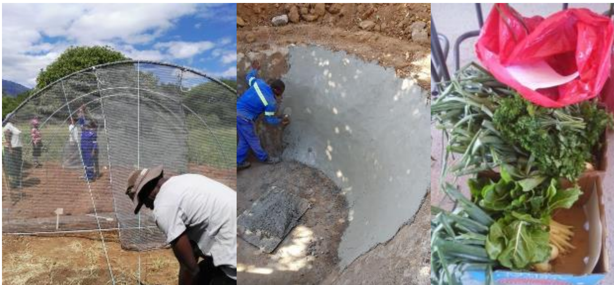
Construction of tunnels (Willows), Underground RWH tanks (Sedawa), Organic marketing (Hoedspruit Hub)
