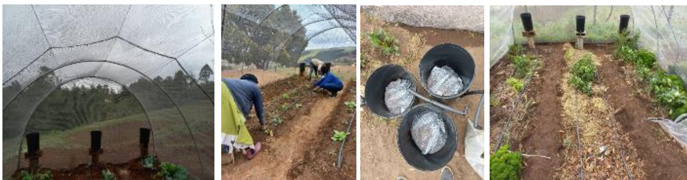
Figure 7: Midlands: Above Left: Drip kits installed in MamZondi's tunnel in Gobizembe, Above centre: Laying out the pipes after putting in the string drippers for Mrs Xulu (Ozwathini) Above Right: Making of the stone and sand filters for the bucket drips for Mrs Mhlongo (Ozwathini) and Above Far Right: Installed drip system for Mrs Chamane's (Ozwathini) mulched beds in her tunnel.
